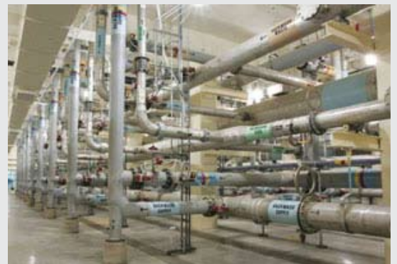
Stainless steel pipe from producer Outokumpu was used in the construction of the Minneapolis water treatment facility.
